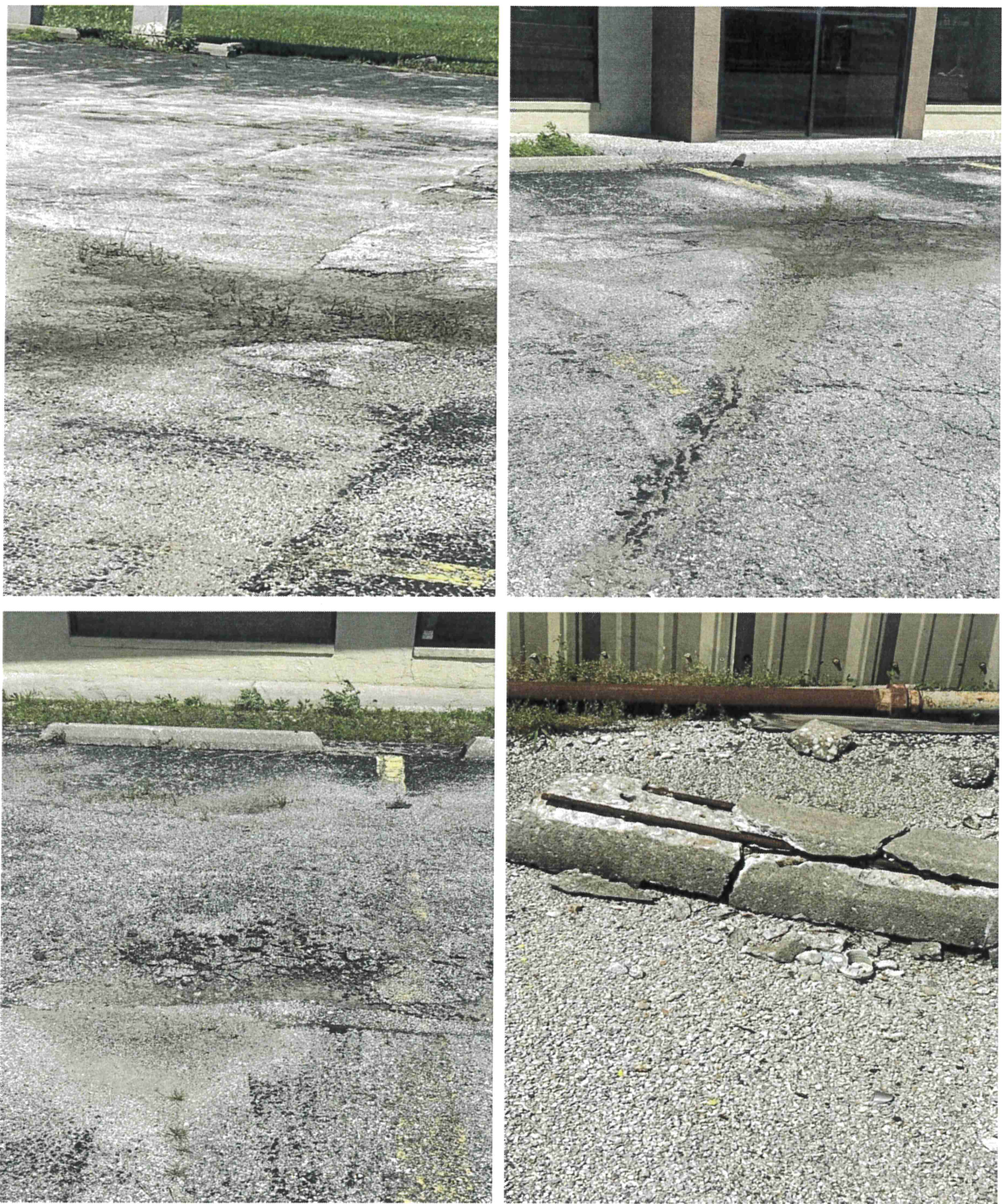
Figure 7: Deteriorated Parking Improvements
