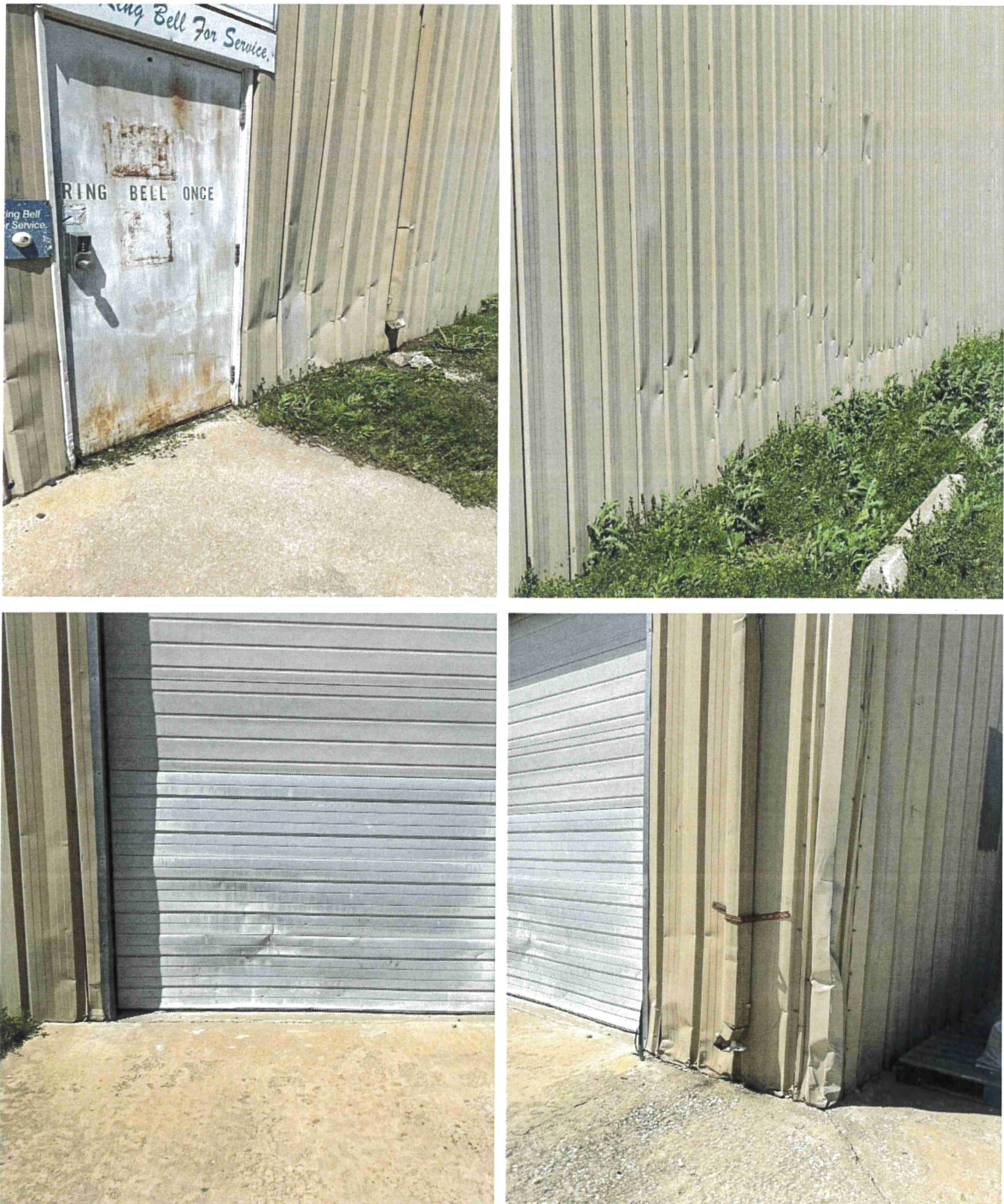
Figure 5: Degradation of Building Exterior
