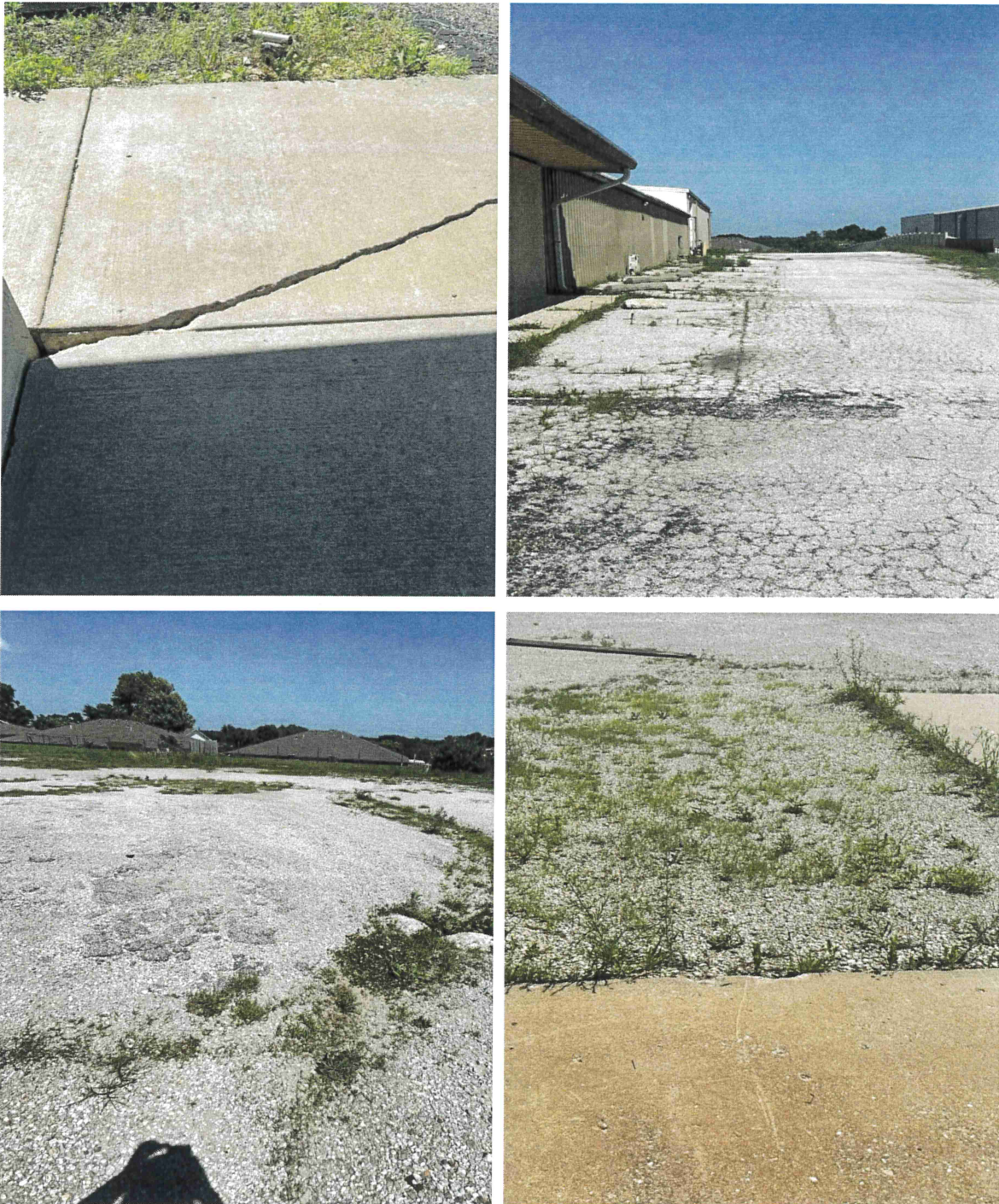
Figure 8: Deteriorated Parking Improvements
